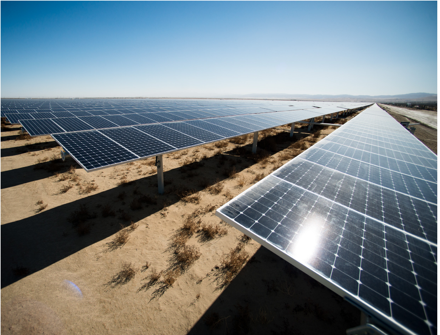
Stanford solar generating station
